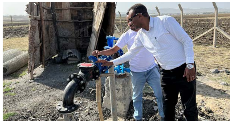
Installed concrete electric poles and installed submersible at the LWF water supply project. © Sophie Gebreyes/LWF. May 2022.
