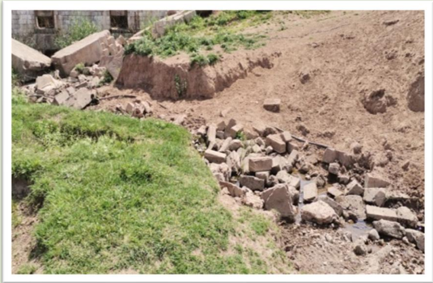
Figure 26: An inlet of a water canal damaged by floods
