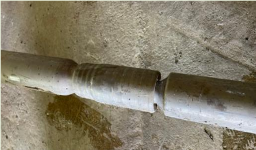
Figure 19: Erosion of the pump flange due to sand.
