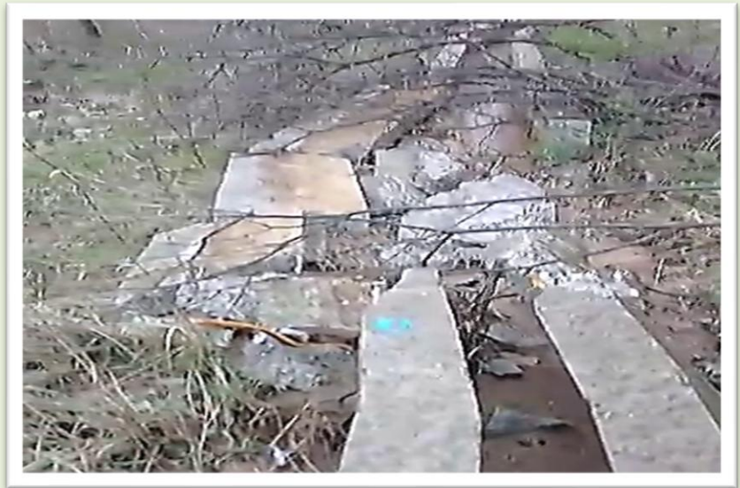
Figure 23: An irrigation canal damaged due to the flood season
